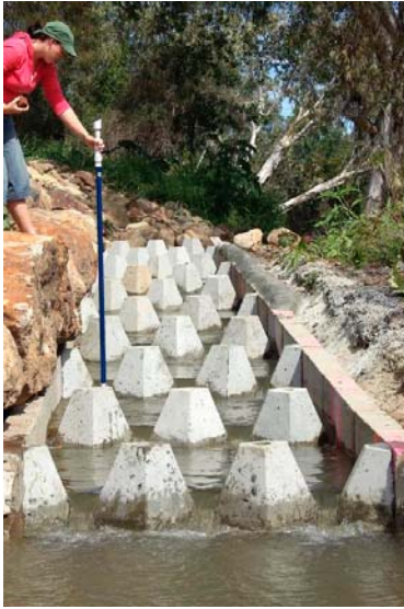
A typical cone fishway installation in Queensland, Australia
