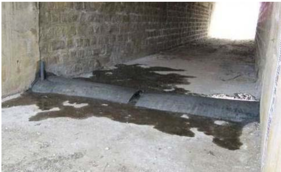
Culvert B weir designed for adequate gauging of flow with minimum impact on users.
