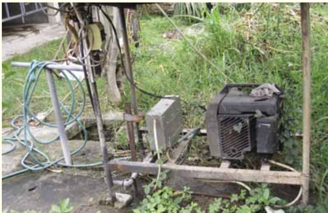
A biogas-driven generator providing electricity for household, farm and neighbourhood use.
