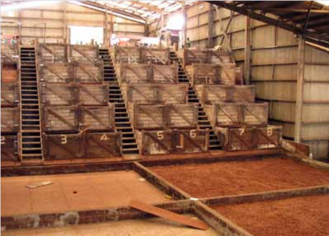
Commercial 'cascade style' fermentary and diesel-fired heated drying beds owned by cocoa buyers and exporters, NGIP-Agmark at Talin, Kokopo. This unit can ferment up to 20 tonnes of wet bean per week. (Photo: Y. Diczbalis)
