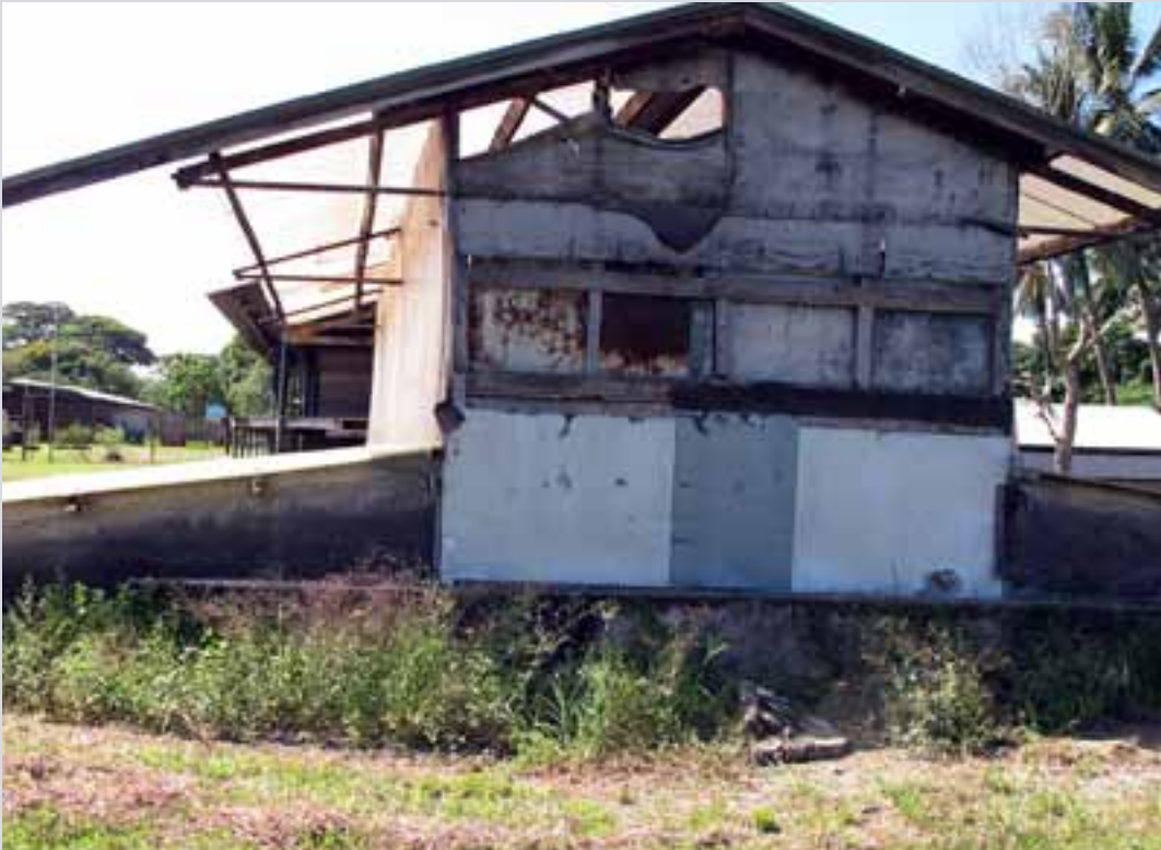
Solar dryer at Vudal University (Keravat Campus) with a 3 m × 10 m drying area, built by the project in 1997, capable of drying 3 tonnes of wet bean at one time. (Photo: Y. Diczbalis)
