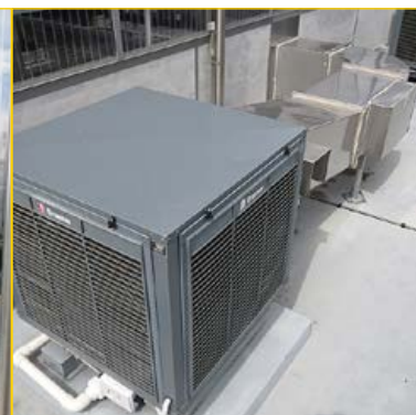
Figure 2.12c Evaporative coolers duct cool air through to the plant house.
