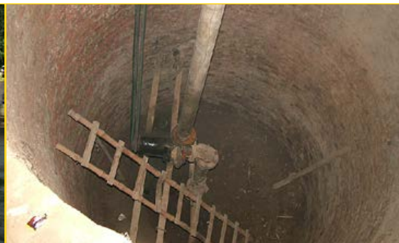
Figure 11.3b Inside a tube well showing the lined wall and pump.
