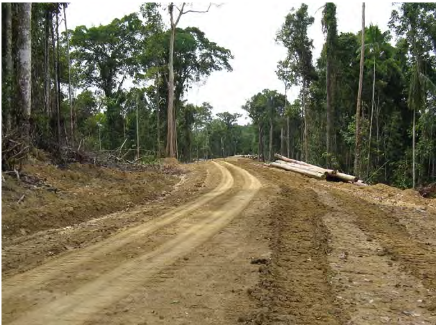
Roads created to access the forest can account for a relatively large proportion of effected area during selective-harvesting operations. Here is a temporary logging road constructed in Western Sepik province (Photo: Joe Pokana).
