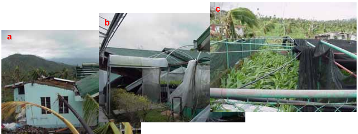
Fig 17. Coconut tissue culture facilities damaged by Typhoon Reming: a) laboratory extension building; b) greenhouse / humidity chamber; c) nursery
