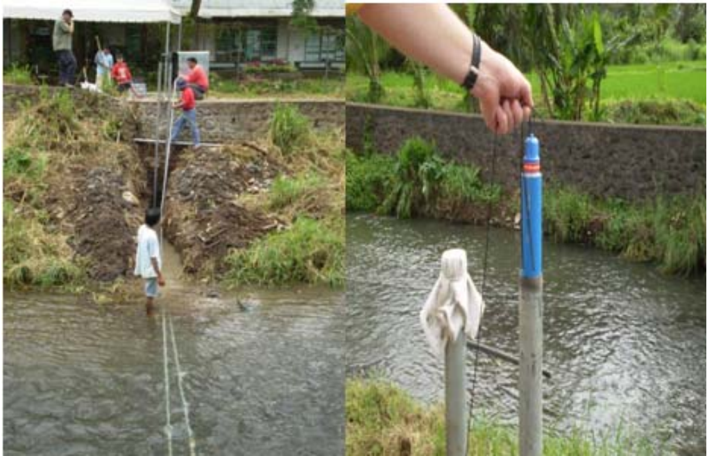
Figures 8 and 9. Installation of the stilling wells for the Odyssey water level loggers and the logger within the well at Lucban.
