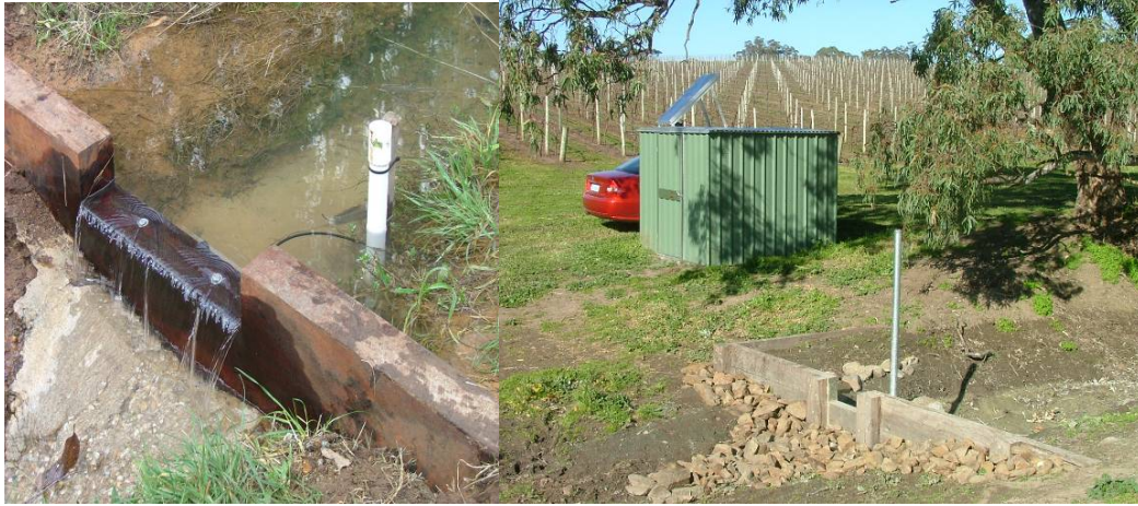
Figure 20. The stilling well for the flow meter bubble line and the rectangular weir at the cherries site.
