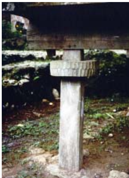
Rat guards fitted to the foundations of a traditional grain store in the Philippines
