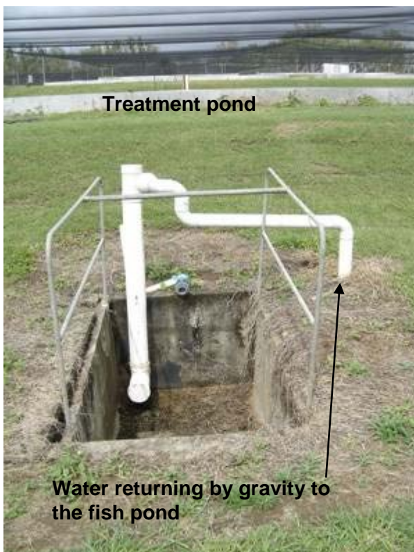
Figure 6. The external stand pipe structure allowing water to overflow from the treatment pond back to the fish pond.
