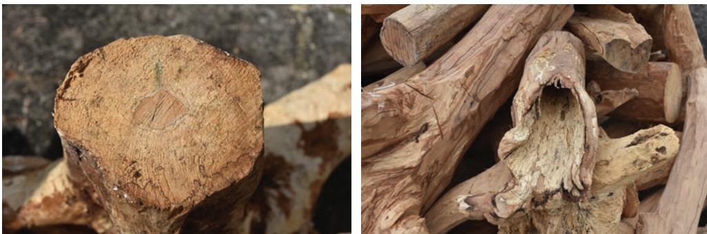
Figure 11.10 Rotten wood – heartwood with significant areas of degradation associated with water or disease entry into the wood
