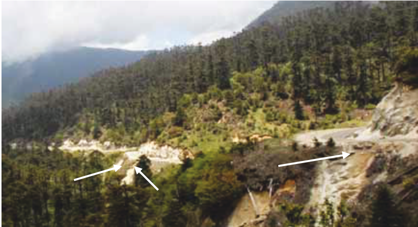
Figure 5 Soil erosion resulting initiated by road construction in sub-alpine forest (see arrows)
