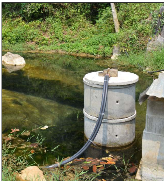
Figure 6: New pump installed on spring at Thong Khang to supply water to the Thong Khang Agroforestry Station (Photographer: Mark Dieters)
