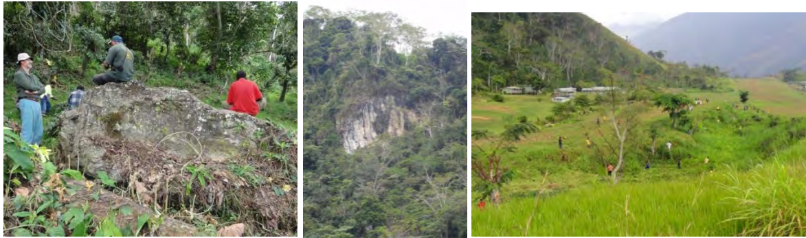
Plate 25 Left - Large blocks of limestone and calcareous sandstone which have fallen from exposed cliffs above (centre). Right - View down the Tapini airfield toward the rim of the landslide, note Primary School buildings on the left. High school students are cutting grass in the stream channel, the stream is piped under airfield and the alluvial soil (ACIAR SP12 was described on the right-hand-side middle-distance of photograph.
