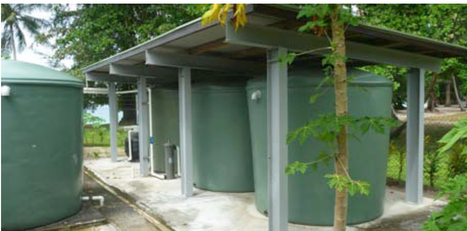
Figure 3. Covered water storage tanks at the mariculture facility on Nago Island, PNG
