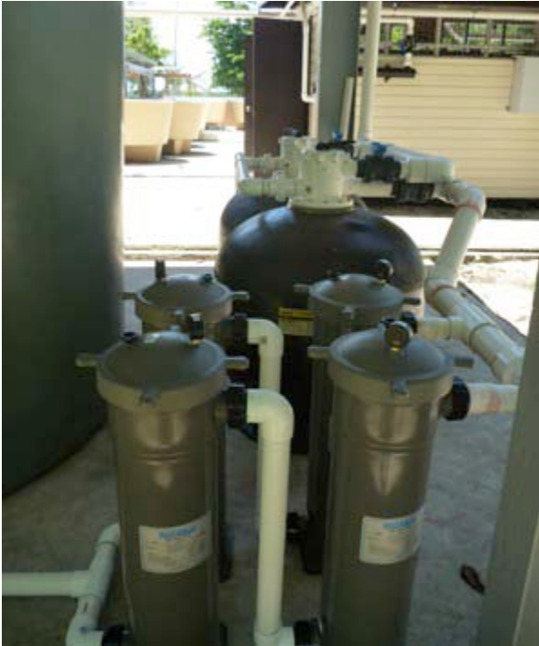
Figure 2. Sand and bag filters
