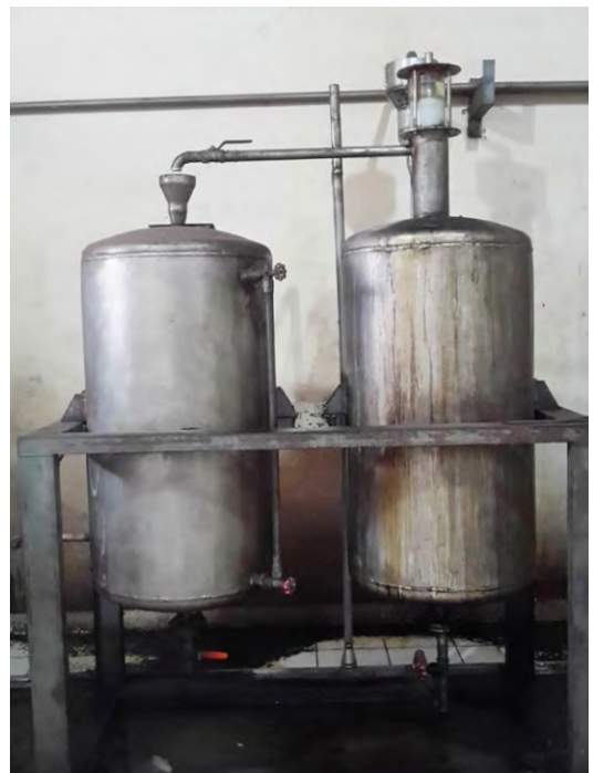
IMAGE 42 Oil separator (right) and collector (left) at Sendangmole cajuput oil distillery, Gunungkidul Credit: Prastyono
