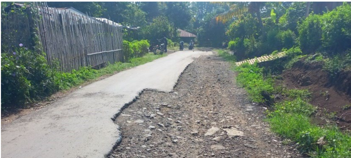
Figure 10 Road condition around North Bajawa Subdistrict
