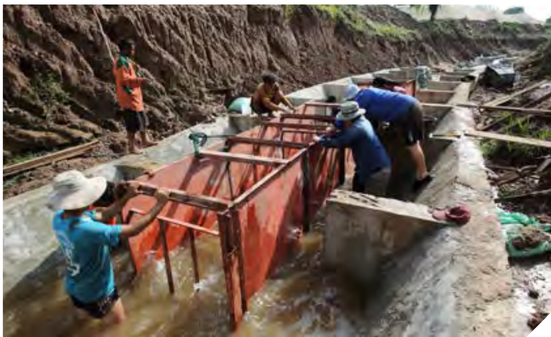
The success of fish passages in Laos, such as this one established beside a dam in Bolikhamxay Province, has led to DFAT support to scale up the technology across the Mekong Delta. Photo: ACIAR | 2012
