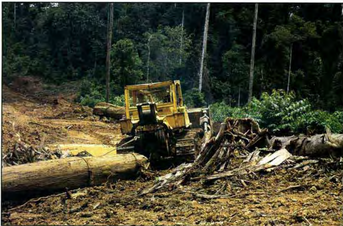
Where heavy machinery is employed during logging, up to 30% of the surface may be bared in roads, log landings and skidder tracks. (Photo: L.A. Bruijnzeel)
