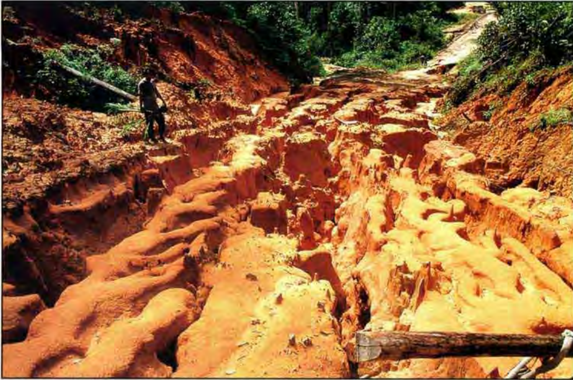
Heavy erosion is often observed on poorly-drained roads, especially where erodible sub-soil is exposed in steep road sections. (Photo: T.C. Whitmore)
